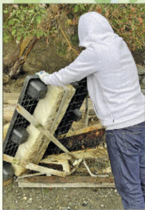
PHOTO COURTESY CLAIRE SICHERTMAN Jeremy Sichertman tries to take apart a piece of an old dock before taking it up the stairs from Baker Beach on Saturday.
