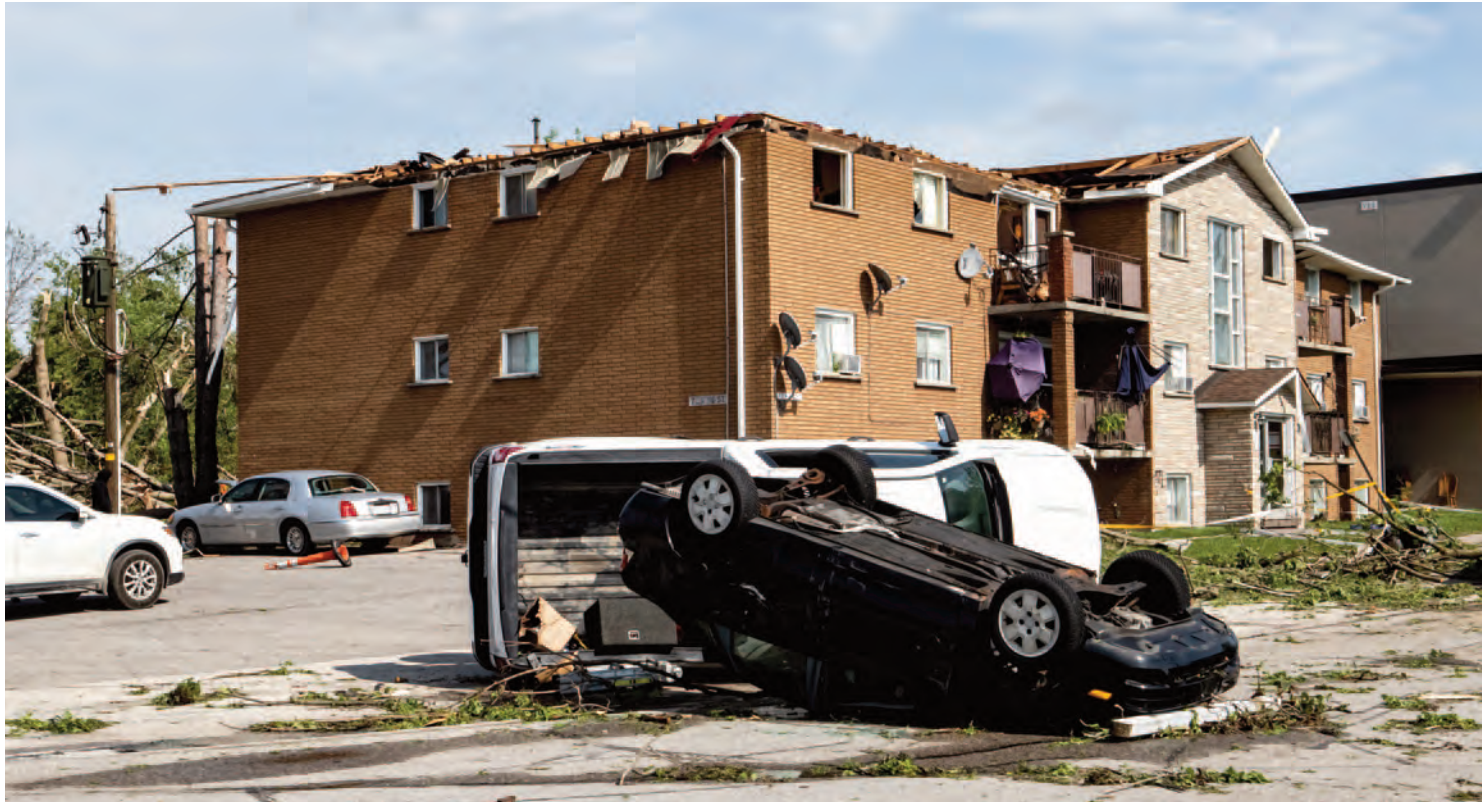
THE AFTERMATH - The unassuming apartment building at the corner of King St. W. and Spruce St. (across from the train station) sustained significant damage when a severe storm ripped through Uxbridge on Saturday afternoon. Dozens of cars were damaged, power lines were cut down by trees, and a state of emergency has been put in place for the entire township. Photo by John Cavers
