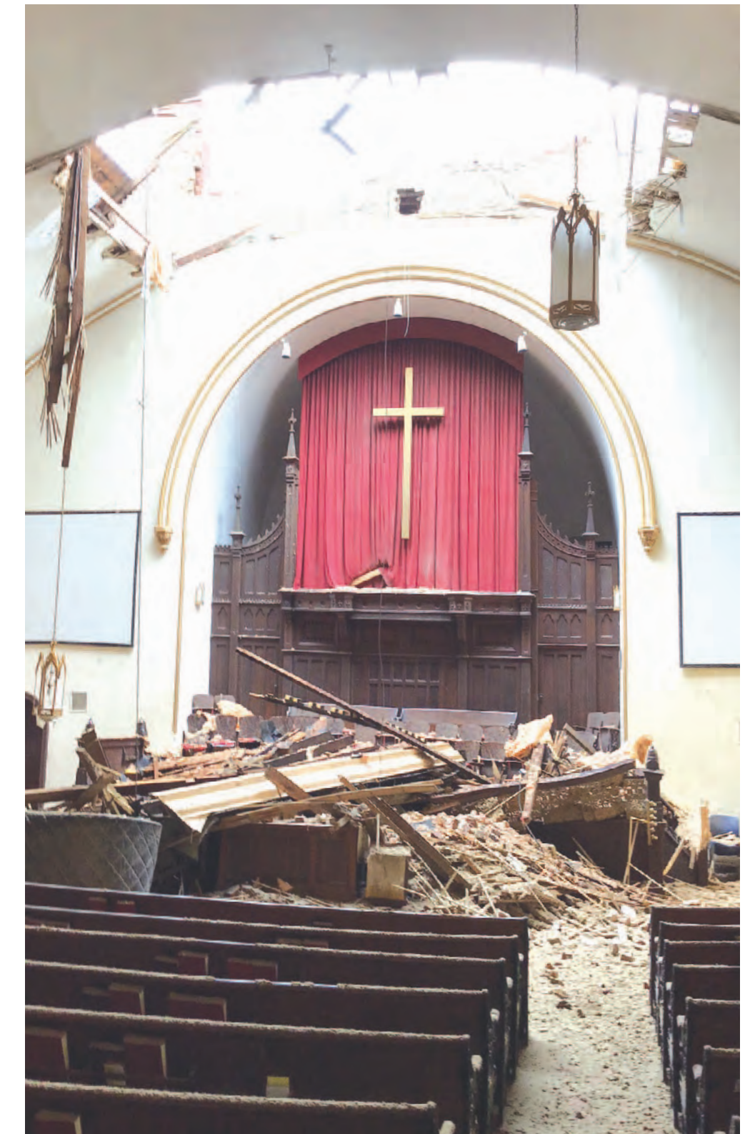
The storm blew the roof off Trinity United Church on First Ave.; debris covers the altar. Photo by Conrad Boyce
